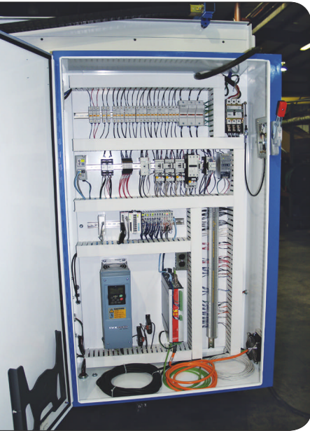
Using EtherCAT and standard Ethernet cabling, Kays Engineering was able to cut two entire work days from the required wiring time of their Eldorado and DeHoff control cabinets.
